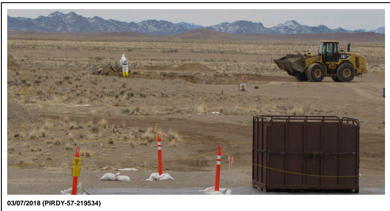
Figure 2-1 SG1, Excavation of Buried Debris in Zone 4 (Zones 1a and 1b in Background) Facing Southeast
