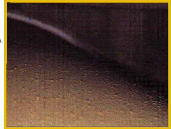
Dust on canister surface at Calvert Cliffs (EPRI 2014)
