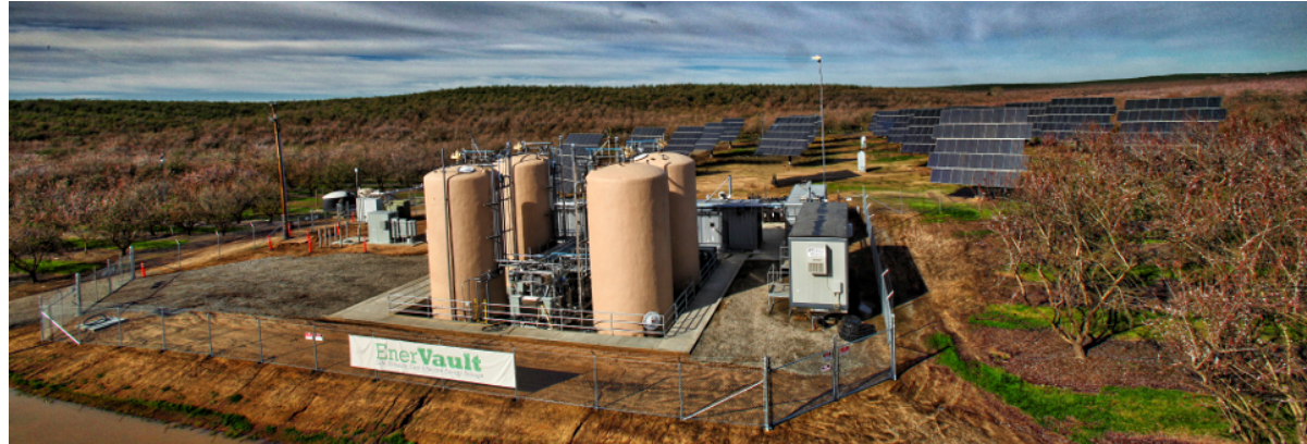
EnergVault plant, Turlock, CA. 250kW, 1 MWh.
