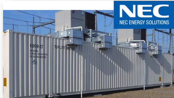
2 MW/3.9 MWh ES System at Sterling Municipal Light Department, Sterling, MA
