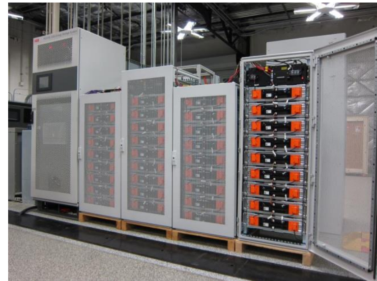
SCE Tehachapi plant, 8MW, 32MWh.
