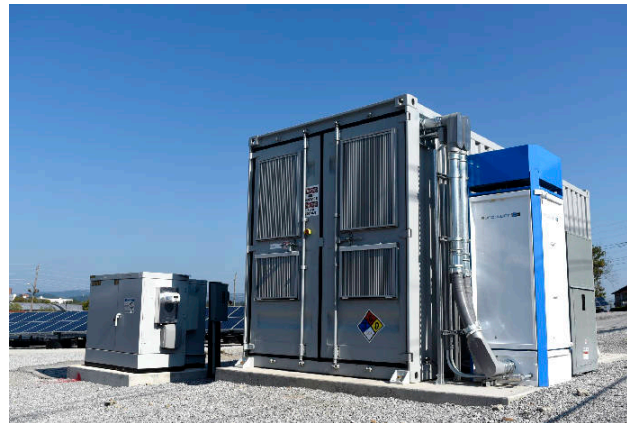
100kW/400kWh Vanadium Redox Flow Battery EPB, Chattanooga, TN
