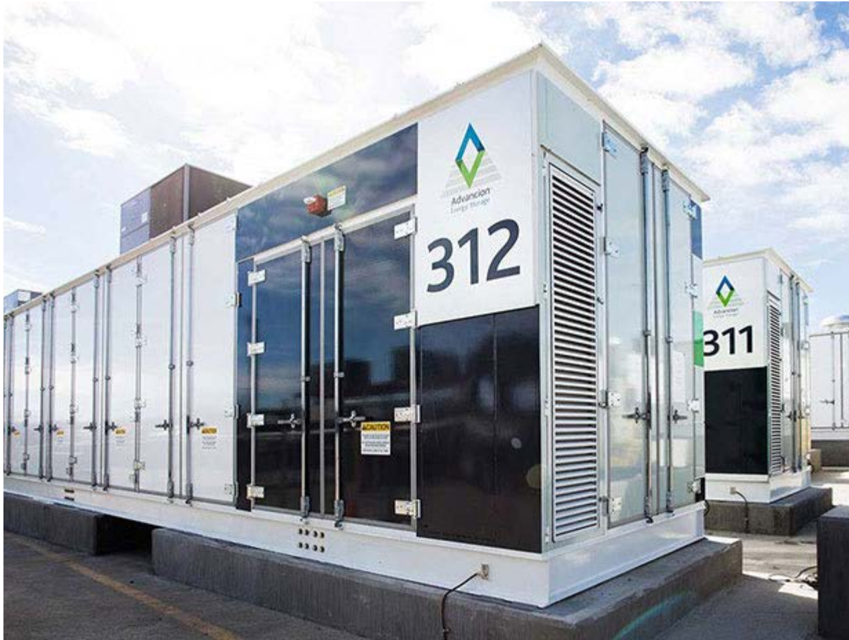
SDG&E 30 MW/120 MWH lithium-ion battery energy storage system in Escondido, Calif.
