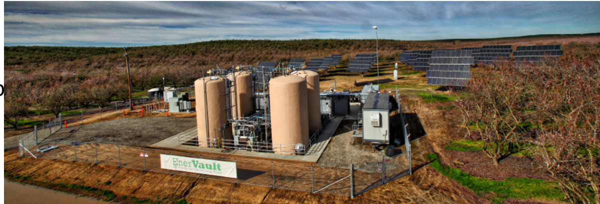
Enervault plant, Turlock, CA. 250kW, 1 MWh.
