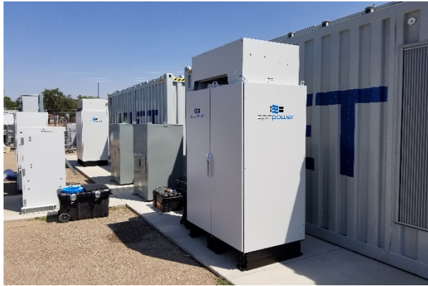
250kW/1MWh UET Reflex flow battery system at Sandia Energy Storage Testpad
