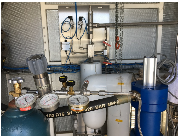
Figure 55: Picture of the setup used on April 20 th 2017 to test the pump
