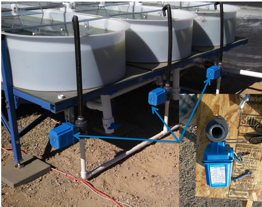
Figure 44: Influent actuated valves.
