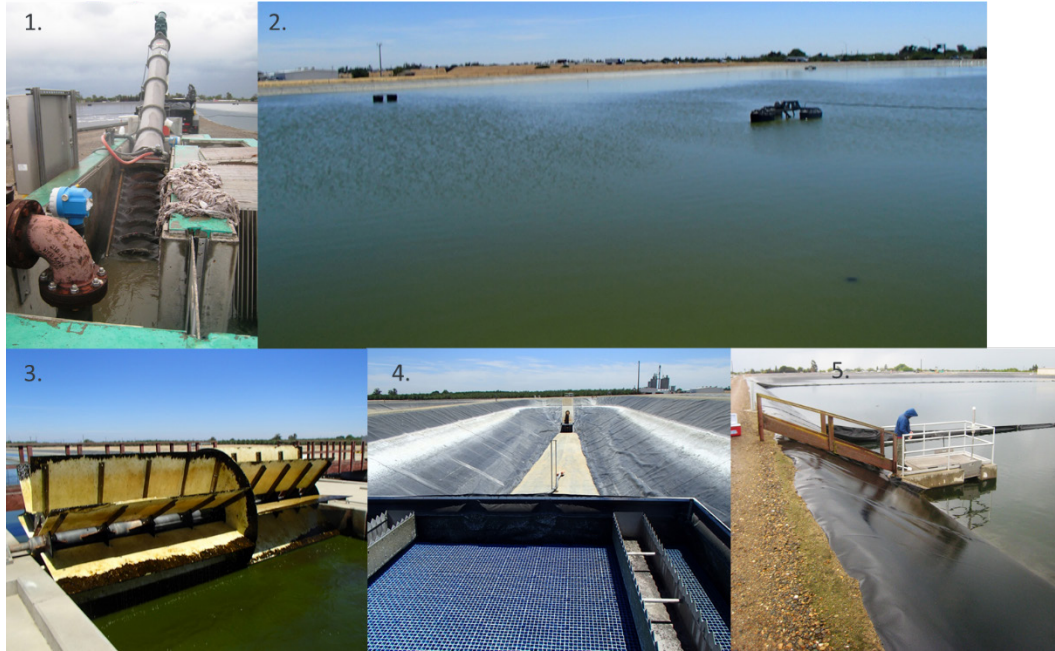
Figure 18: Major unit processes at the Delhi wastewater treatment plant including (1) the influent bar and rotary screen (2) a facultative pond with a floating aerator (FAC), (3) the paddle wheels of the high-rate ponds (HRAP), (4) an empty algae settling pond (ASP) and (5) the maturation pond (MP).
