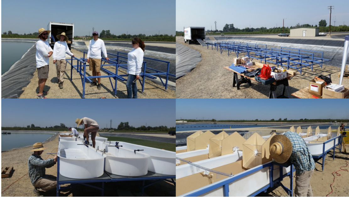
Figure 43: Installation of the pilot ponds started with the construction of the frames. Then the ponds and center baffles were installed. Finally, the paddle wheels were added.
