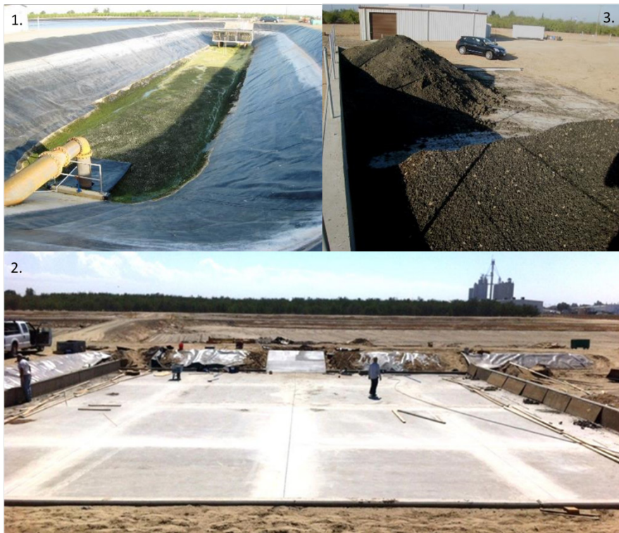
Figure 19: Solids handling at the Delhi wastewater treatment plant including (1) Decanting the algae settling pond (2) the concrete drying bed, (3) and piles of solar dried biomass.
