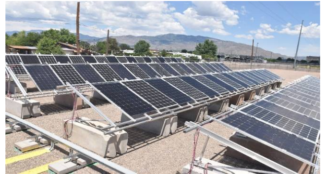
Fig. 9. Sandia's fixed-tilt string-level arrays, Albuquerque, NM.
