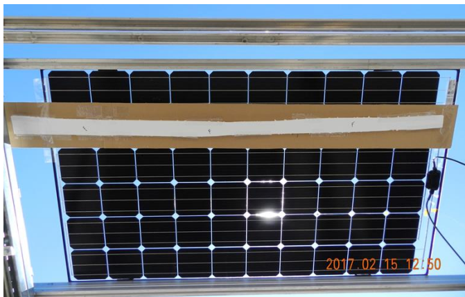
Fig. 3. The obstruction behind a bifacial PV module in "direction B" with 20% coverage. Obstruction is in contact with the rear surface of the PV.
