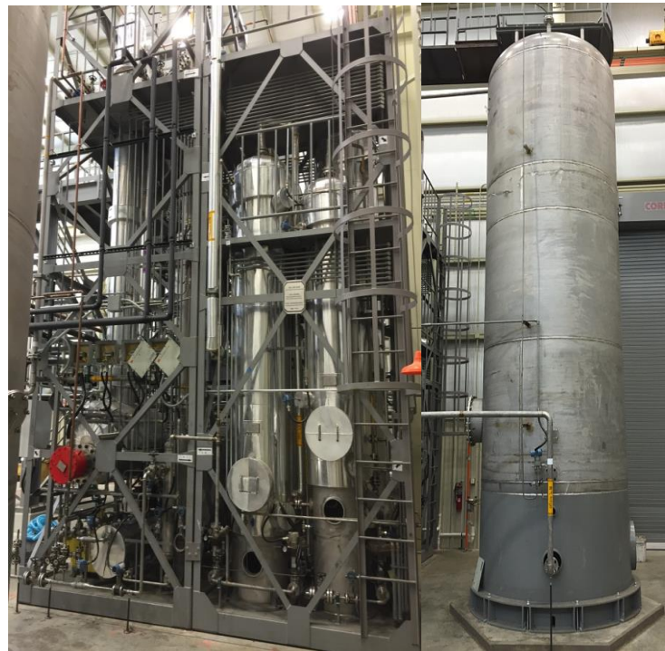
Figure 8: Photo - Acid Gas Removal Unit (left) and Activated Carbon Bed (right)
