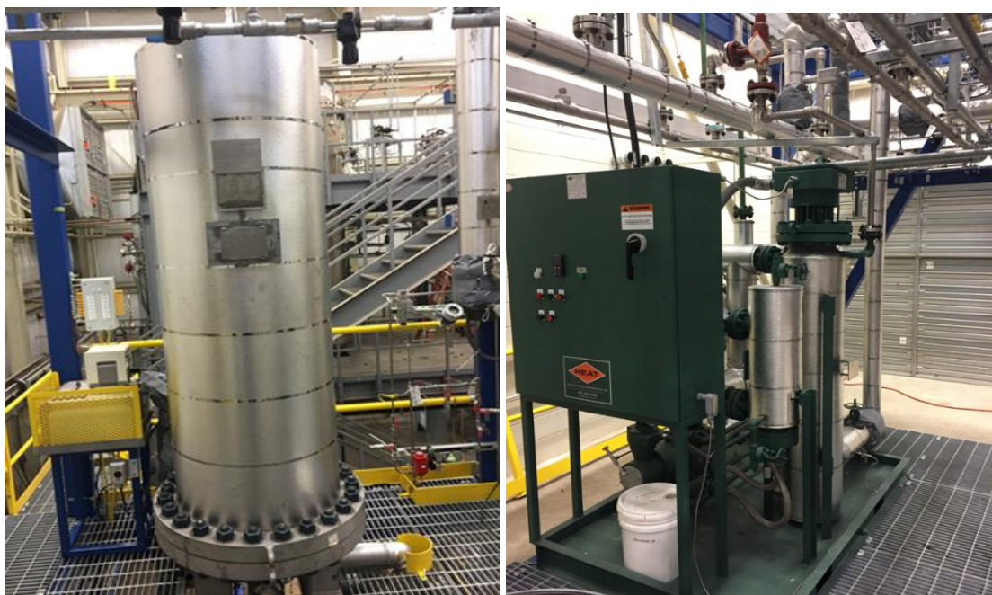
Figure 9: Photo of F-T Reactor (left) and Pressurized Hot Oil System (right)
