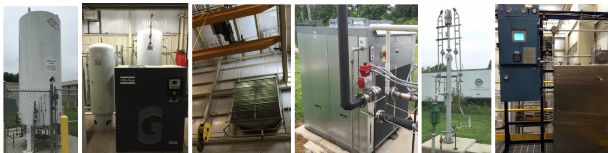
Figure 11: BOP systems (Left to Right): Oxygen Gas, Nitrogen Generator and Air Compressor, Crane, Chiller, Flare and Gas Chromatograph
