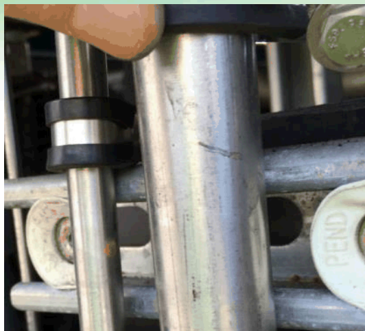
Stainless steel piping under rubber clamp
