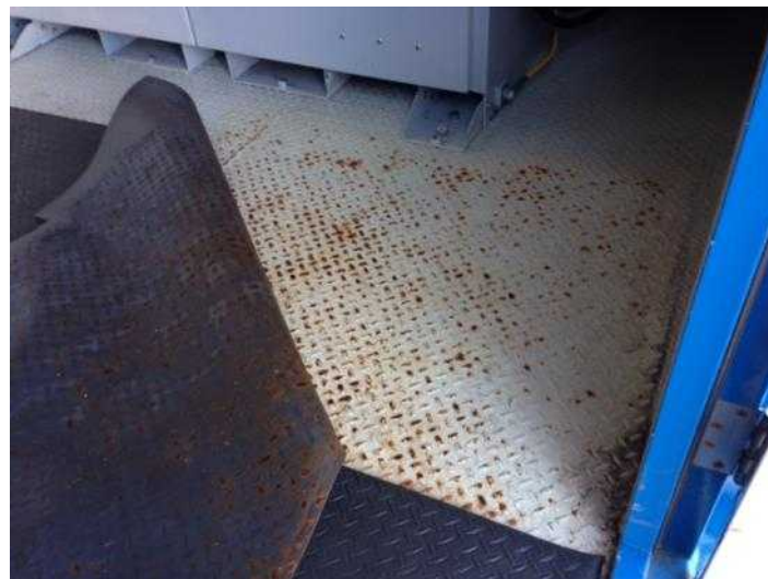
Painted carbon steel floor with trapped moisture
