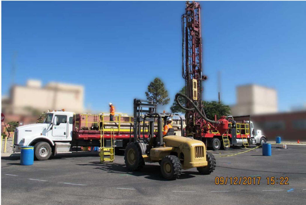
Figure 2-1 The Pipe Truck, Drill Rig, and Forklift on Location for Injection Well TAV-INJ1 in the Technical Area-V Main Courtyard (view to the east, September 12, 2017)
