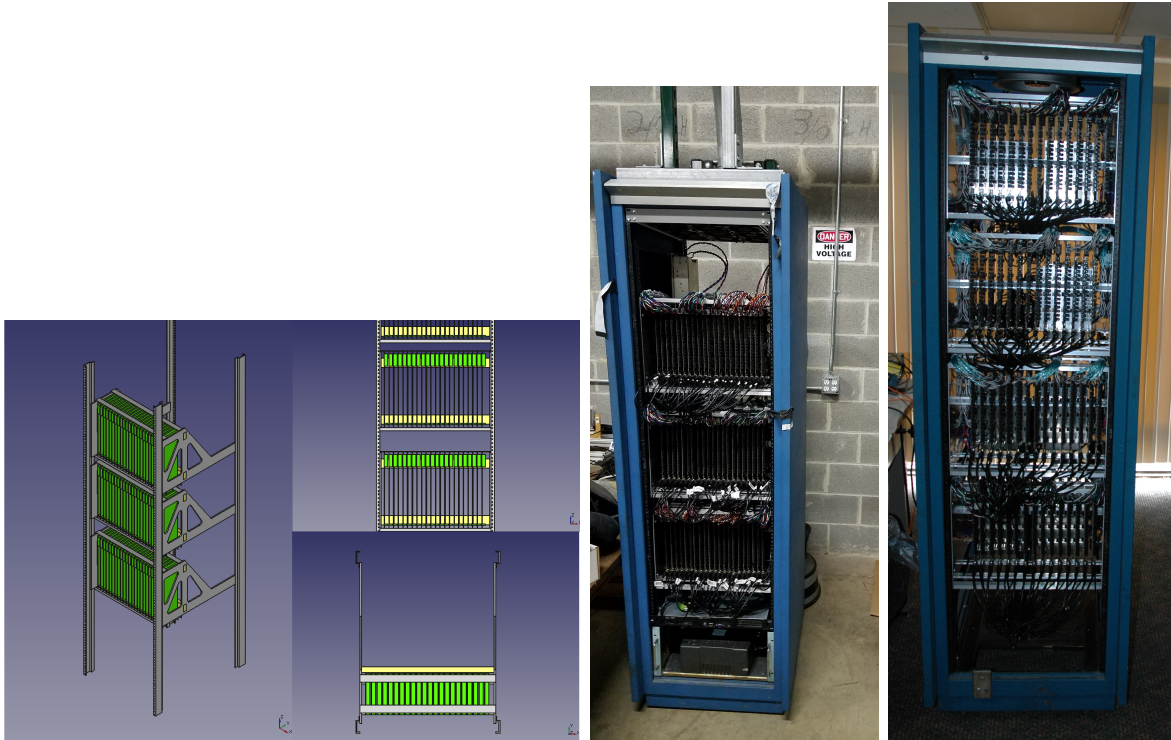
Figure 2 (Left) Emphasis was placed on designs that would allow boards for 1024 photodiode channels to fit into a single standard electronics rack, which assisted in keeping the system electrically shielded and portable. At 16 channels per daughter card, 64 daughter cards would allow 1024 channels. Two cameras were designed and constructed. Camera 1 (Center) used three racks of 21 boards to have 1008 pixels and Camera 2 (Right) employed four racks of 16 boards for 1024 pixels. (The two racks are actually the same height.)
