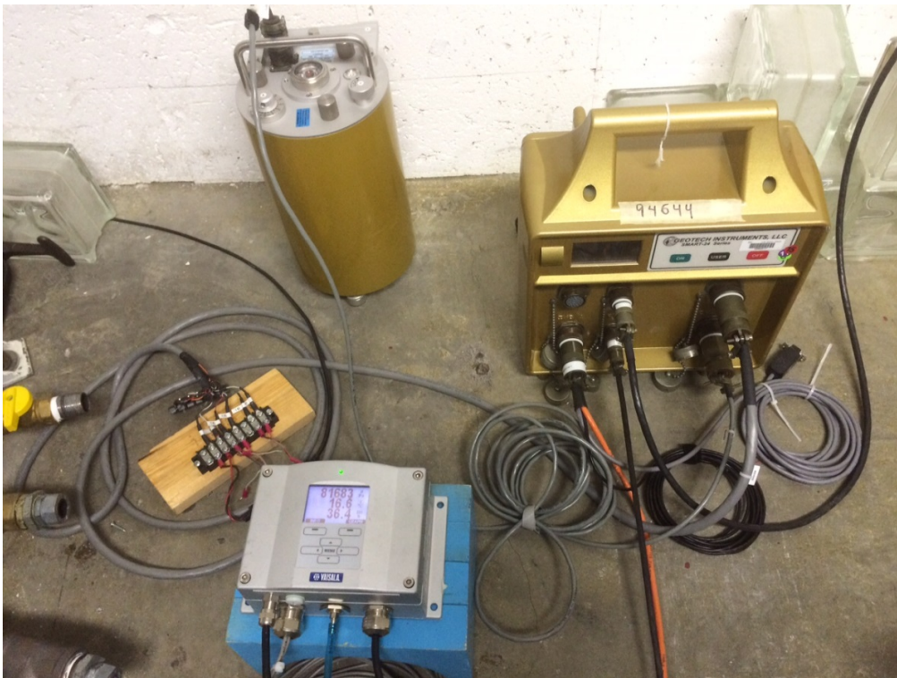
Figure 4 GS13 seismometer and Vaisala pressure & temperature reference
