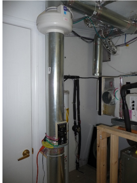
Figure 2-5. Mechanical ventilation supplied to the utility room
