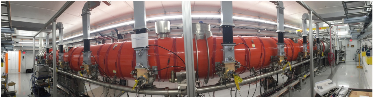
Figure 1: pCM installed in CMTS1 and readied for powering.
