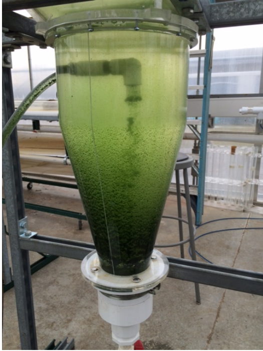
Figure 60. Lamella thickener during initial stage of operation
