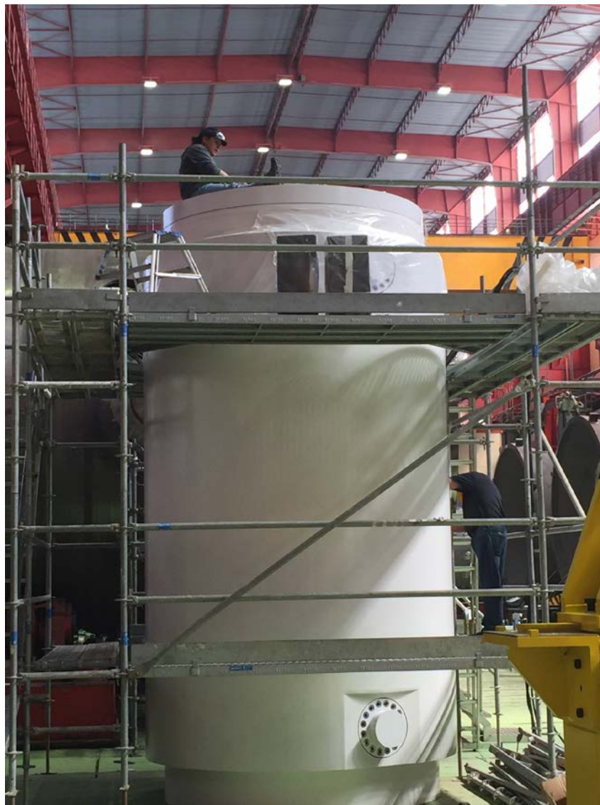
Figure 3-35. SNL instrumentation specialists threading cables into recesses on the instrumentation lid (top) and attaching accelerometers cable along length of cask (bottom).
