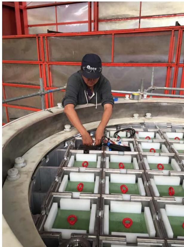
Figure 3-16. Sandia instrumentation specialist gathering assembly instrumentation cables to be passed through instrumentation lid.
