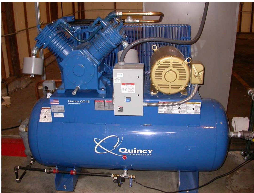
Figure 49 Facility air compressor
