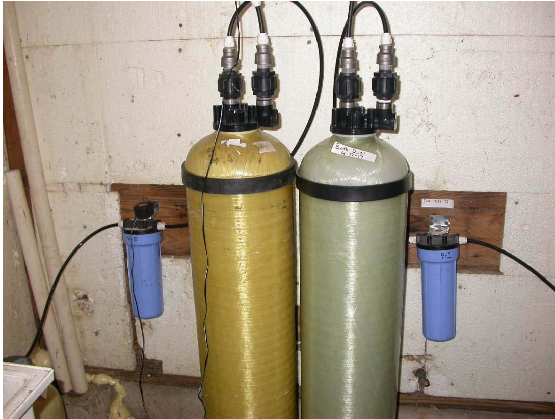
Figure 46 Cartridge filter and resin tanks for deionization system
