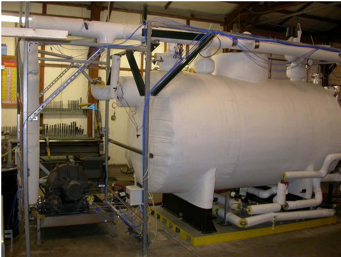
Figure 48 Feedwater storage tank and turbine
