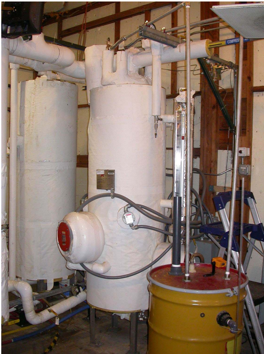
Figure 47 Steam generator and blowdown drum
