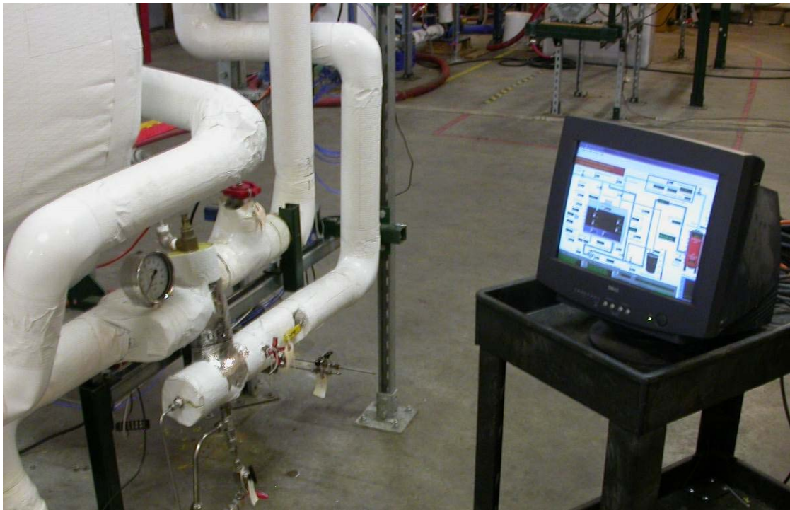
Figure 52 Water injection control station
