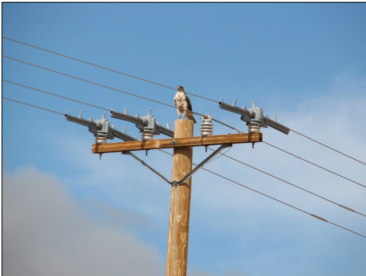
Figure 6-2. Retrofit pole with insulator caps and a red-tailed hawk perched on top of the pole.
