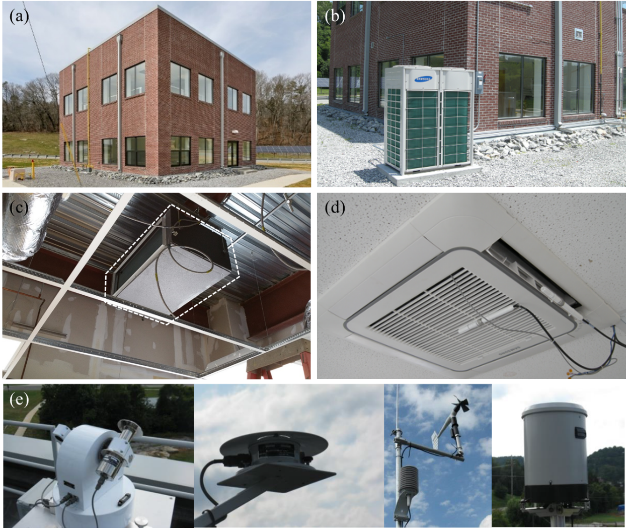
Figure 1. The test facility: (a) two-story flexible research platform, (b) VRF outdoor unit, (c) DOAS unit, (d) one of VRF indoor units, and (e) dedicated weather station on the FRP.
