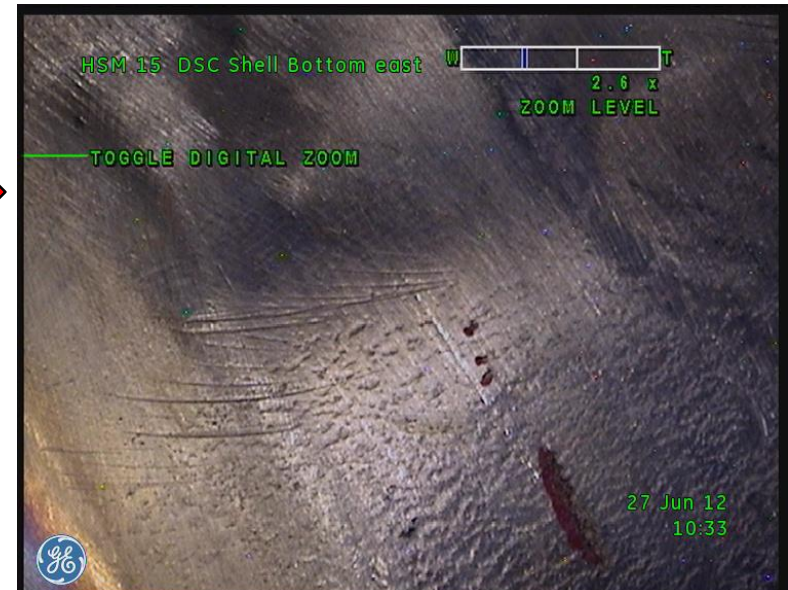
Rust spots on storage canister at Calvert Cliffs
