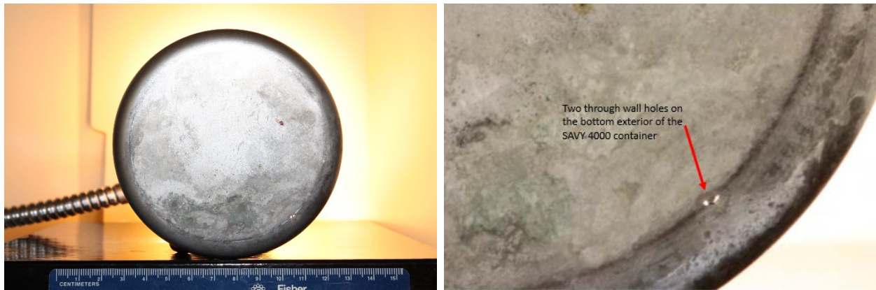
Figure 16 Photographs of the bottom of the SAVY 4000 container after 47 hours of exposure to boiling MgCl_2 .
