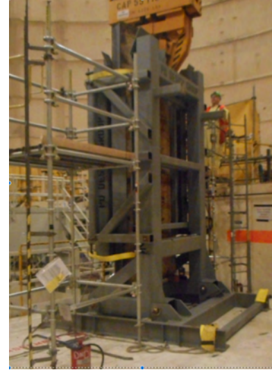
Fig. 5. Gripper crane and “down-ender” frame for repositioning segments into the shipment box [15].
