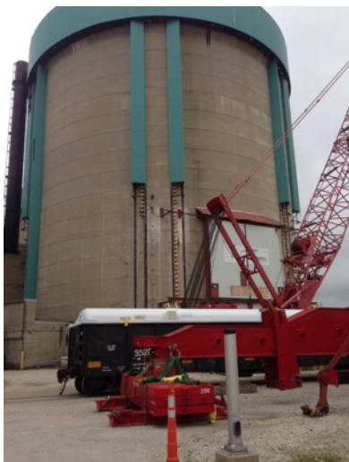
Fig. 9. Crane for loading 2 steel shipping boxes holding 2 pairs of Zion Unit 1 RPV segments into the railcar that was transported to the Memphis Processing Facility [15].
