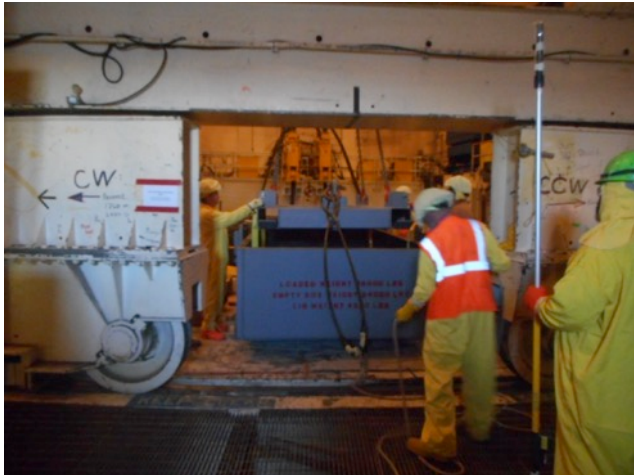
Fig. 8. Closing the steel box containing opposite side segment pairs for shielding and eventual loading into the rail car [15].
