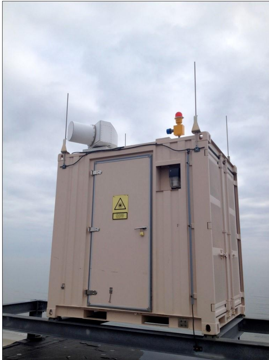
Figure 4. WindTracer instrument shed located on top of Margate Towers Condominiums
