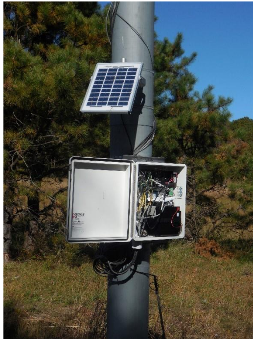
Figure 19. Campbell Scientific CR1000 logger installed at the ACUA mast
