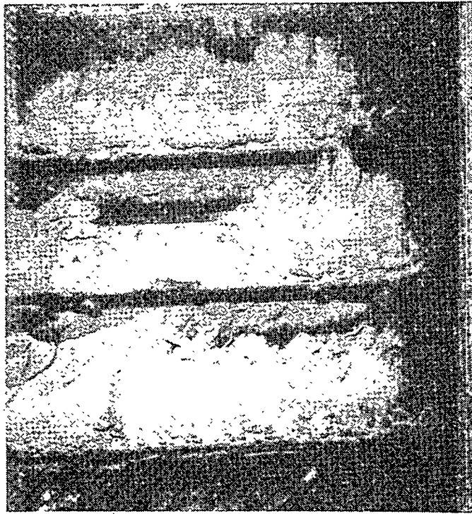
BOILER SUPERHEATER AFTER FIRING WITHOUT LIMESTONE
