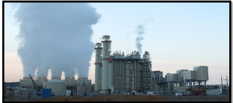
Lake Side natural gas turbine power station in Vineyard, Utah. (Wikipedia Commons)
