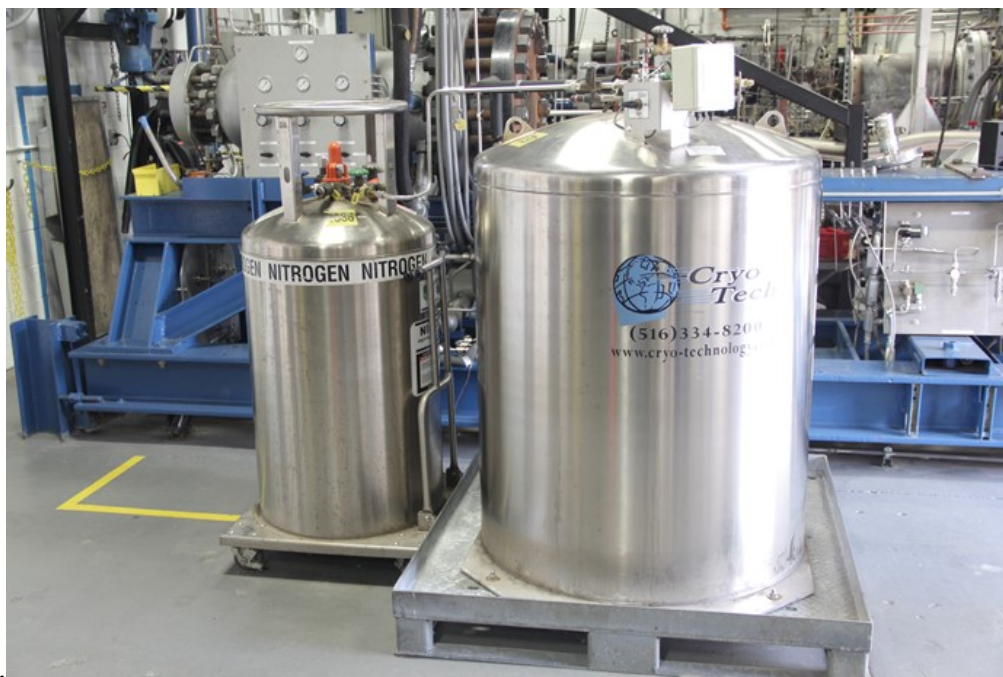
Figure 74: LN2 storage/supply dewars.
