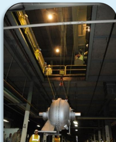
Equipment is lowered from the cell floor to the staging area of the X-326 Building for shipment.
