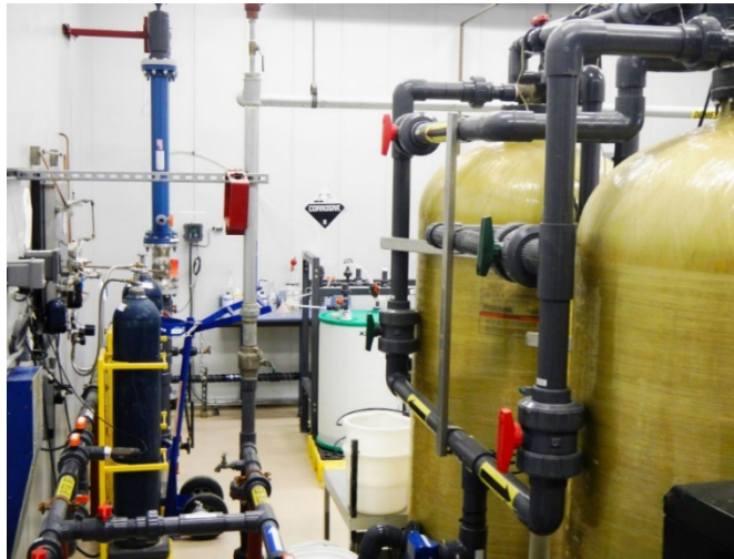
Figure 3-7. SNL/TTR water treatment facility arsenic removal system
