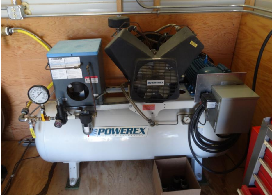
Figure 54. CTRL-145 Compressor and Output
