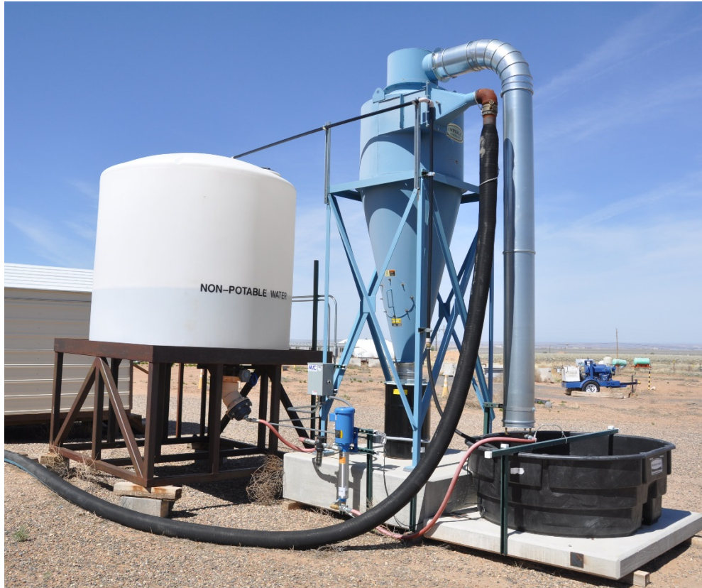
Figure 81. Dust washdown system
