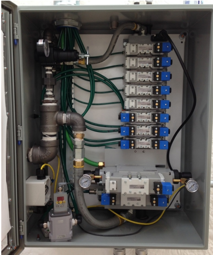
Figure 58. Pneumatic control box
