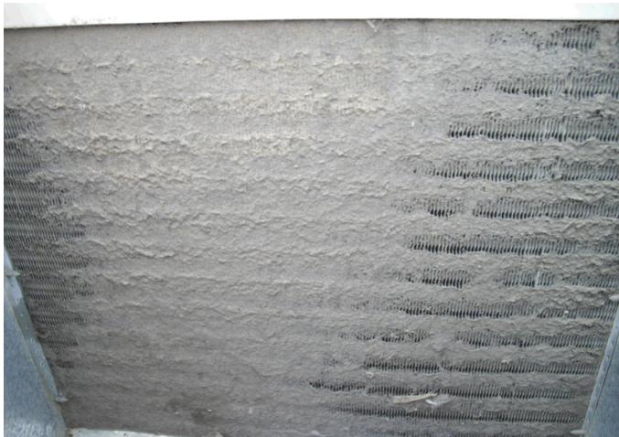
Fouling of evaporator coil 3
