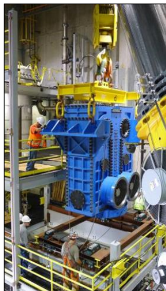
Figure 5. 400 TPD AR dry solids pump installed at EERC
