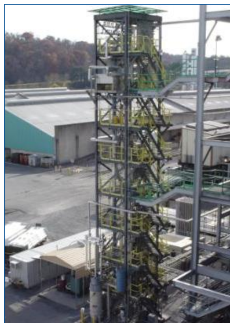
Figure 6. RTI warm syngas cleanup pilot plant systems at Eastman
