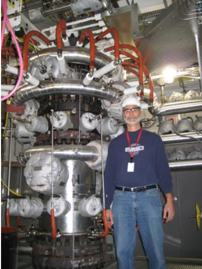
Figure 2. AR compact gasifier system at GTI
