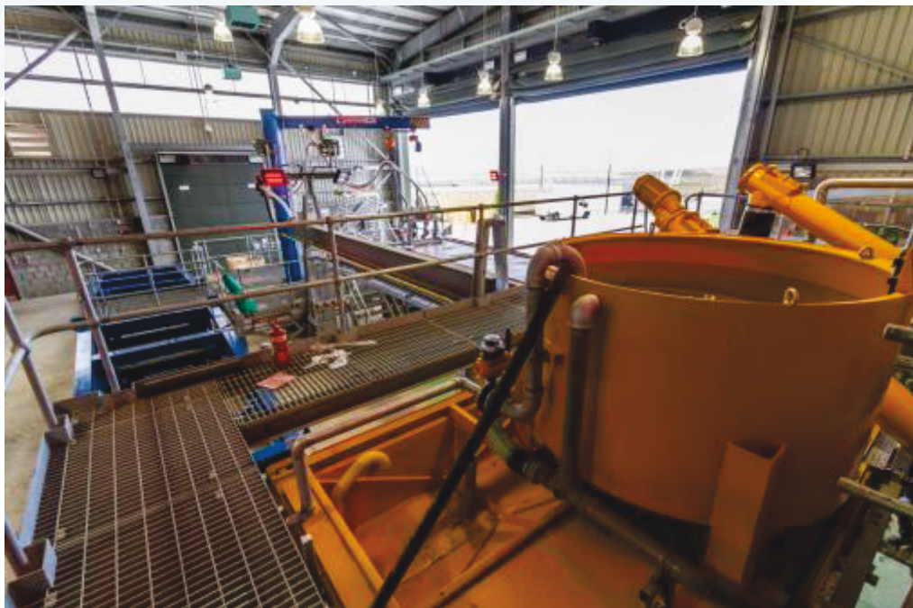
Figure 22. Photograph of the Inside of the Dounreay Encapsulation Plant, Showing the Top of the Grout Mixing Batch Equipment (Ref 253).
