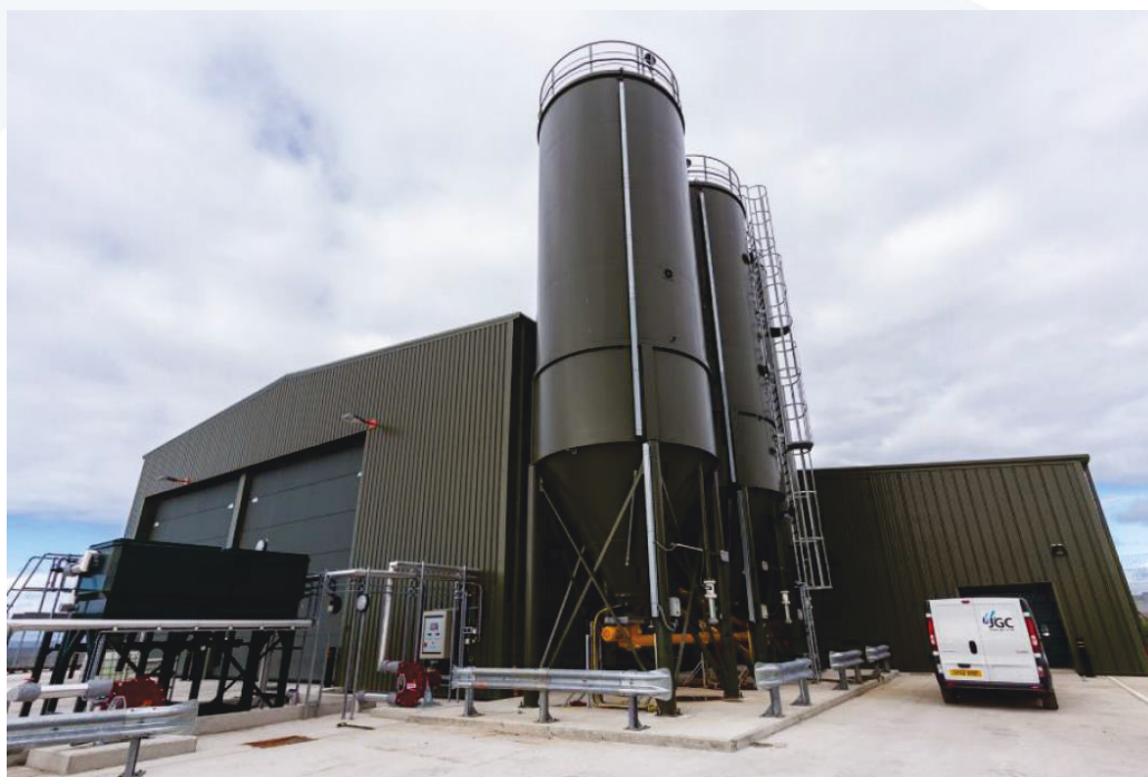
Figure 20. Photograph of the Encapsulation Plant at Dounreay. Silos Contain Dry Grout Materials (Ref 249).
