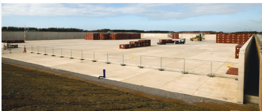
Figure 37. The Recently Opened Vault 9 at the LLWR (Ref 262).
