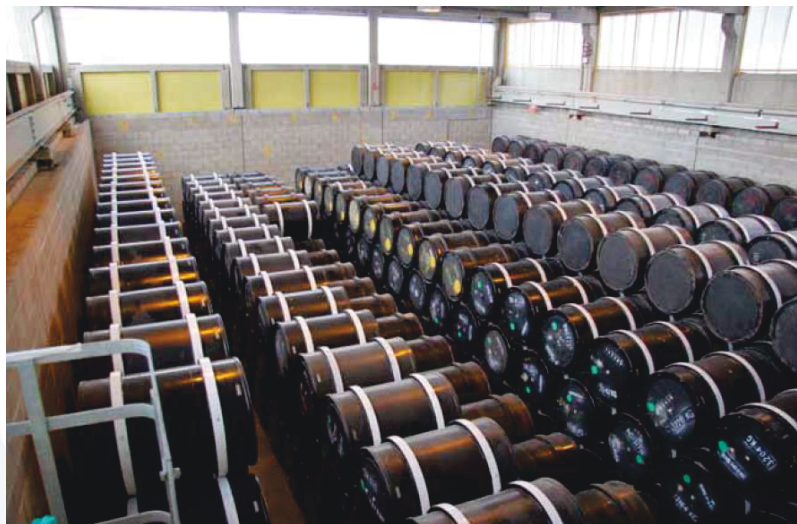
Figure 52. Polymer Encapsulated Resin Drums in Interim Storage at the Shutdown Trawsfynydd Magnox site.
