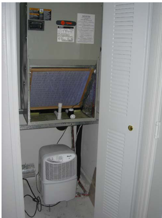
Figure 20. Dehumidifier—Located in return closet
