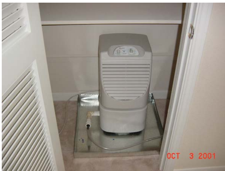
Figure 21. Dehumidifier—Located in closet with louvered door
