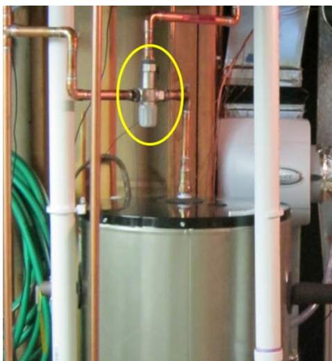
Figure 7. DHW mixing valve
