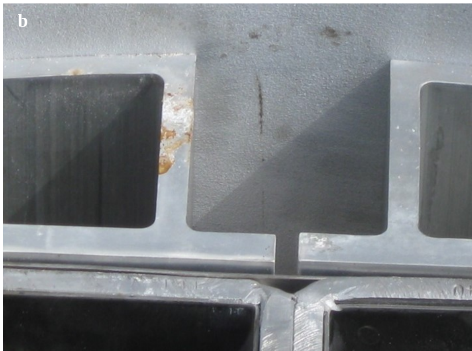
Figure 2. Photographs of a) the “debris” on the basket rail (near side), and b) the “residue” on the basket rail (far side).
