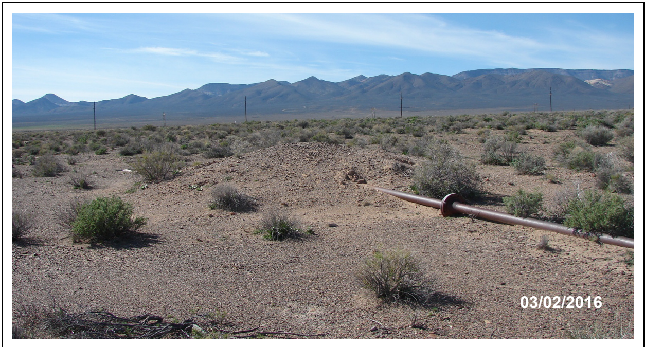
Figure 2-10 SG2: CAS 02-99-12, U2af (Kennebec) Surface Rad-Chem Piping, Pipe (exhaust) Terminating at Soil Mound
