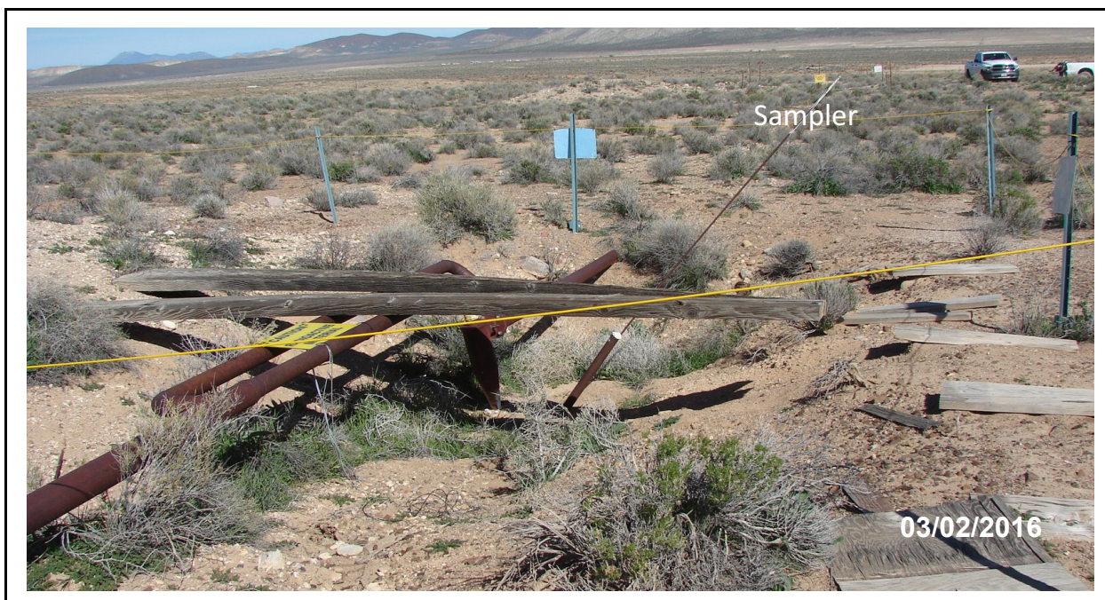
Figure 2-8 SG2: CAS 02-99-12 U2af (Kennebec) Surface Rad-Chem Piping, Sampler at the Sampling Assembly Note: Photograph looking north.
