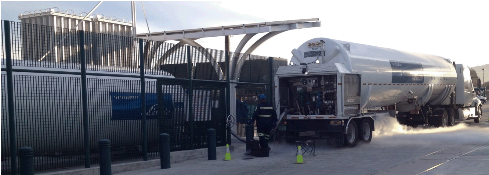
LH 2 refueling at A.C. Transit Emeryville CA hydrogen station
