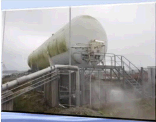
(1) Shoreside storage tank (or refuel directly from truck).
