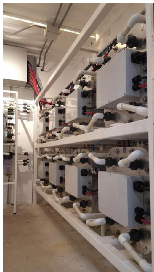
Figure 1. Photo of ESS battery stacks
