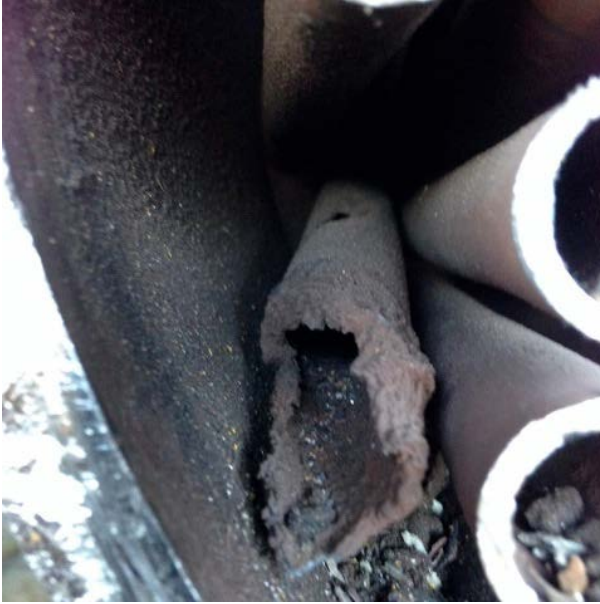
E-120 Tubes after Failure
