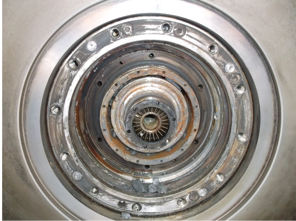
Failed seal on second stage of the syngas compressor.
