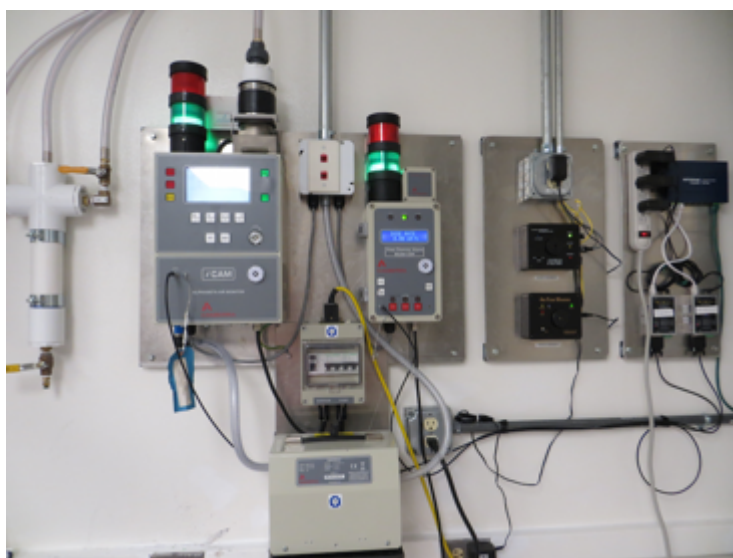
Figure 3. The radiochemistry room counts with a Canberra iCam and Area Gamma Alarm Monitor G64 connected to Ethernet and alarm systems. Data from these instruments is recorded 24/7, year round. The airflow alarms are also connected in case the airflow becomes limited or obstructed. Air exhaust is sampled by the Canberra iCam monitor at approximately 30 L/min using a method 5 isokinetic probe. The isokinetic probe was installed at the center-line of the exhaust duct for the a) Hot Cell (500 cfm) and the b) the Biosafety Cabinet (1100 cfm).
