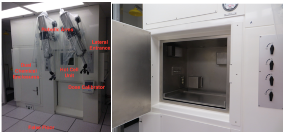
Figure 4. Hot cell with dual chemical enclosures for the chemical separation of Zn-62/Cu-62. The target is manually transported to the facility for further processing.
