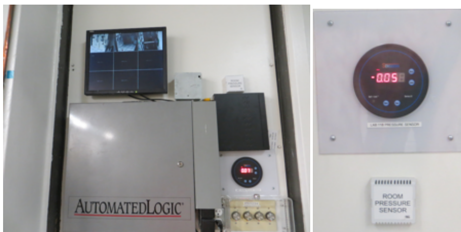
Figure 2. Room pressure and airflow is controlled using an automated logic-board to assess changes in airflow from the room and anteroom, hot cell and radiochemical fume hood. The room was classified as Clean Room ISO 7.
