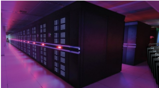
Tianhe-2 (National SuperComputer Center in Guangzhou) Intel Xeon E5-2692+ Intel Xeon Phi
