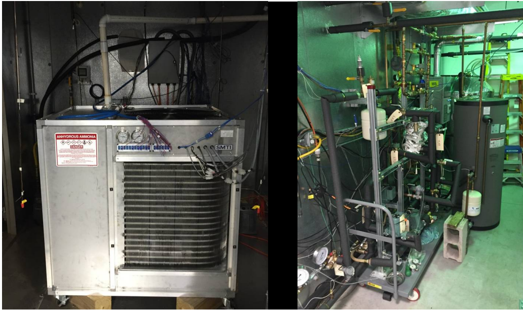
Figure 42: Photos of GAHP within Chamber (L) and External Boiler/Primary Loop (R)
