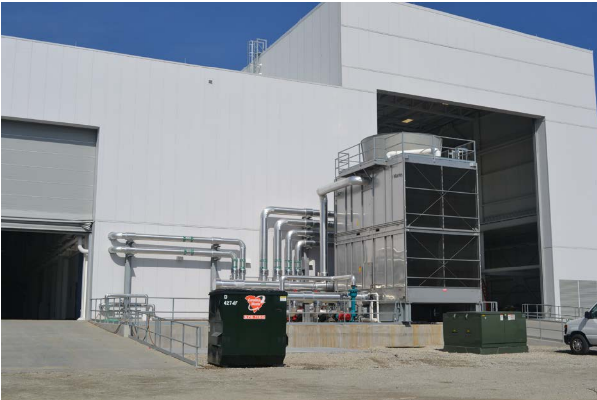
Figure 29 Installed 1500 Ton Cooling Tower
