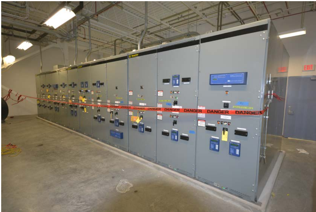
Figure 25 Main Facility 23.9 KV Switchgear
