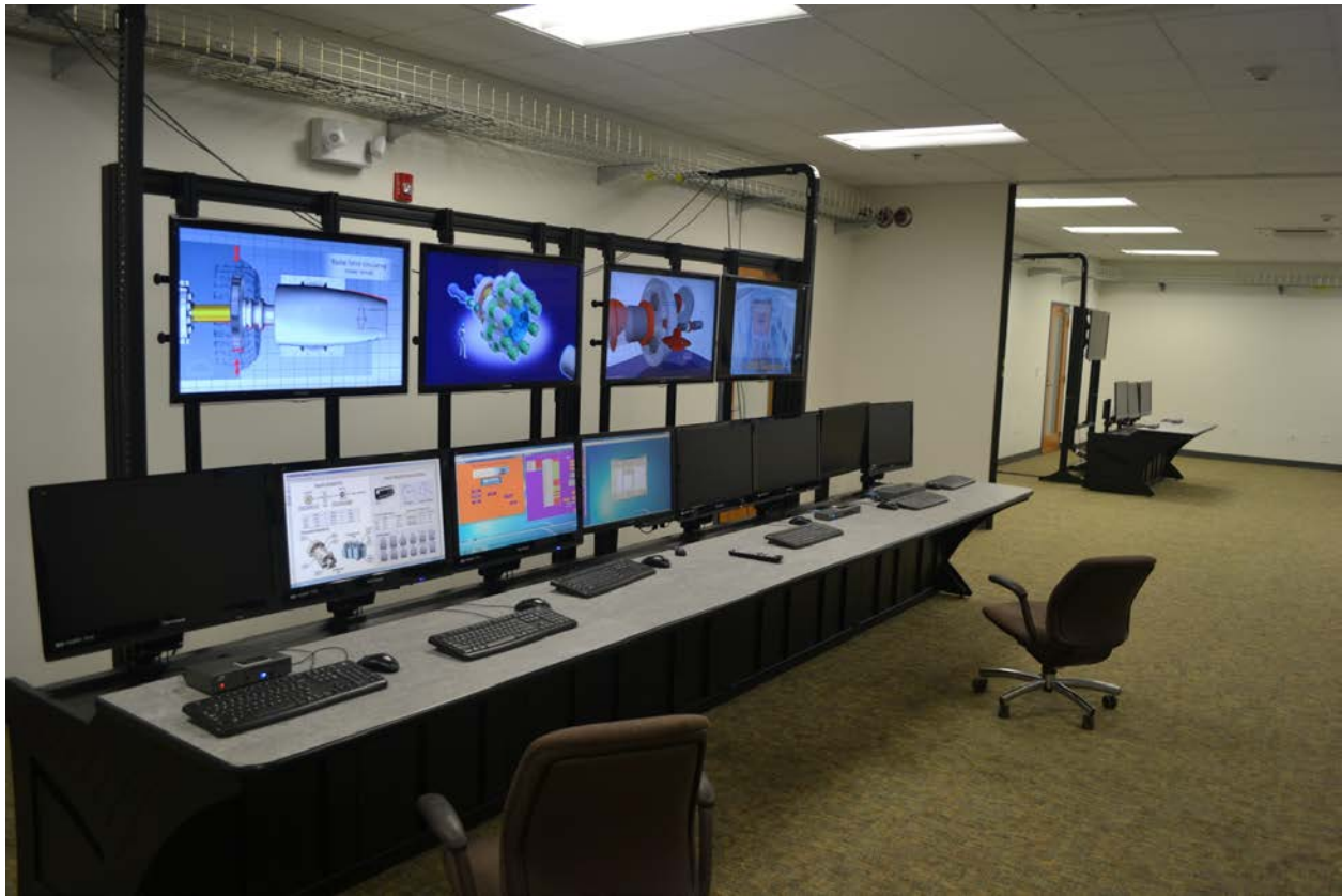
Figure 28 Control Room Console
