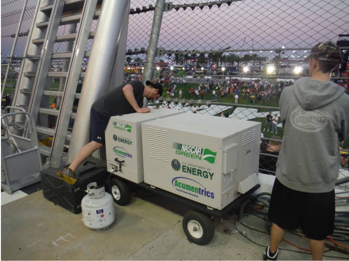
Figure 12 Grandstand Location of 1000 Watt Unit
