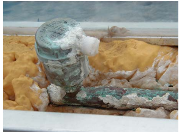
Figure 11. Vent valve showing the effects of a long-term leak through the valve.
