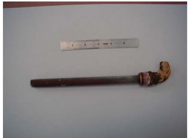
Figure 13. Inlet into tank from the solar absorber.
