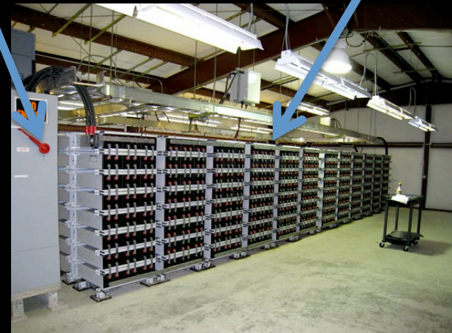
Lead acid Alaska facility designed to replace back- up diesel
