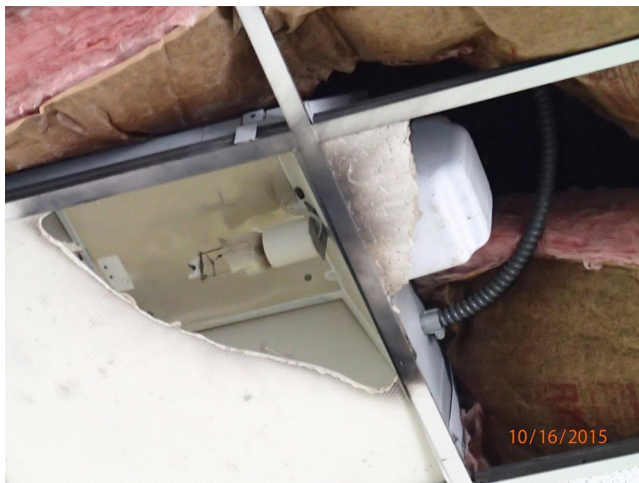
Figure 5. Metal-halide lamp position.
