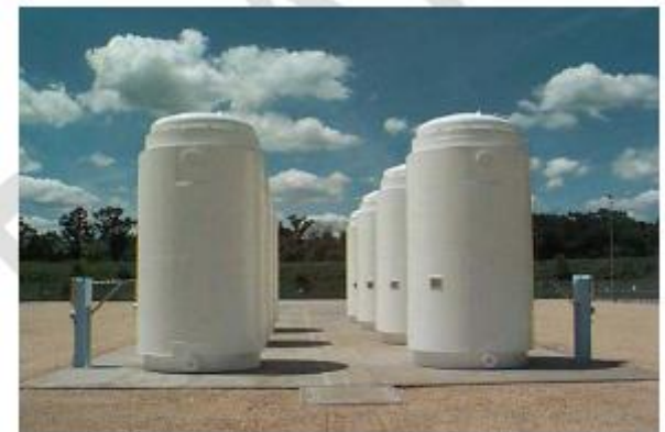
TN Metal Dry Storage Casks.
