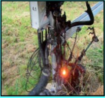
Arcing at the combiner box.
